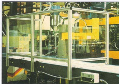
Guard Mounted to Conveyor System and Machine
